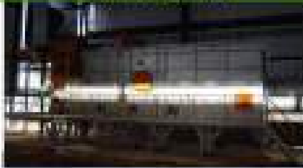
dryer furnace - chip burning
