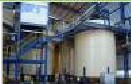
Mixing and Cooking Tanks
