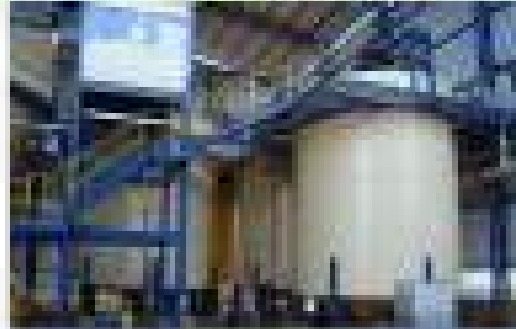
Mixing and Cooking Tanks
